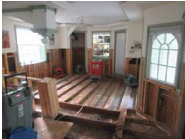
Figure 32. False (Raised) Floor
